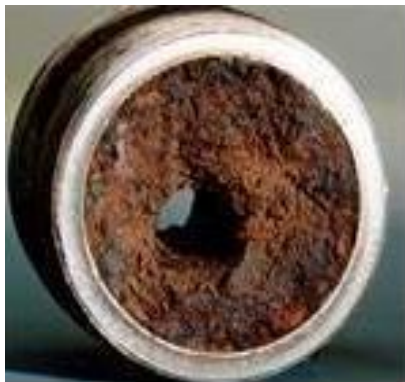
Typical paraffin clogged pipe
