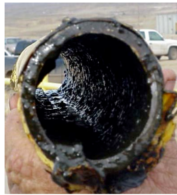
Pipe after SpiroFlo
